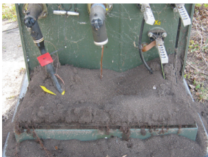
Massive earthen build-up in the transformer
